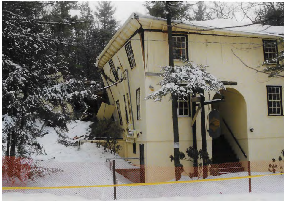
Above: The front (Pennsylvania Avenue) portion of the Playhouse after the auditorium roof collapse.
